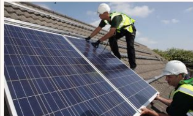
Workers install solar panels on a property in Cornwall. Over the last decade, the costs of solar energy have fallen 89%. Photograph: Simon Burt/PA
